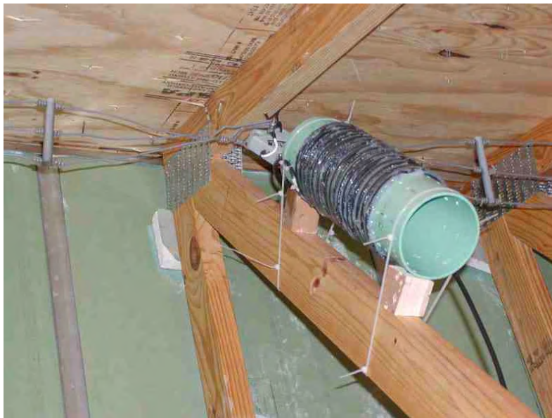
The Dirty Balun and 3 Wire Installed in Attic of the Harvey Villa
