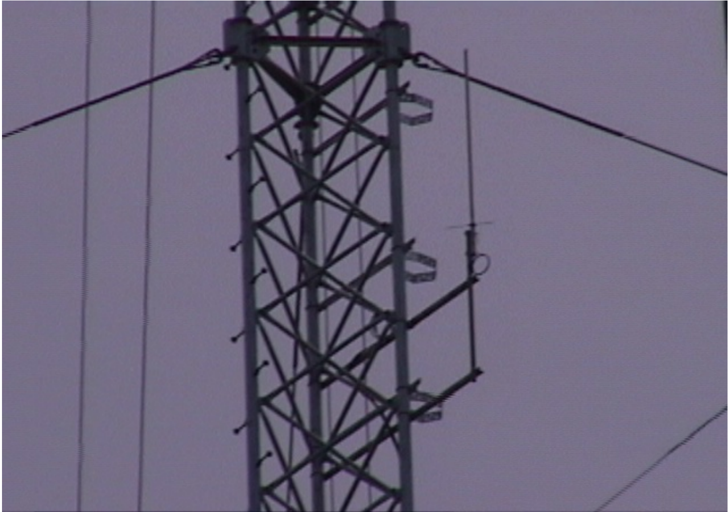
Current WTRA RACES Combined Packet Node and Remote Base Antenna 150 foot level, Receive / Transmit
